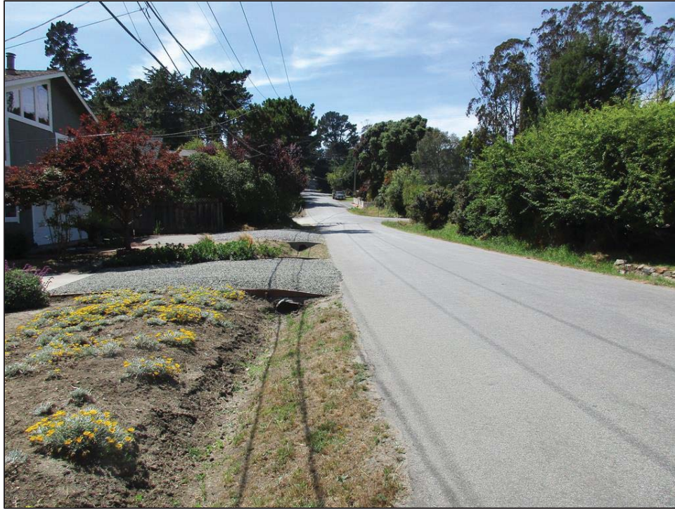
Photo 5: View looking west along Harte Avenue showing the roadside drainage ditch and series of culverts conveying water toward the unnamed creek.
