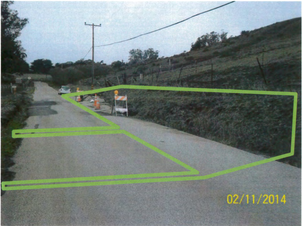
Photo 1. – Photo of landslide damage on Lobitos Creek Cut-off looking west. Marsh Ranch is north of Lobitos Creek Cut-off. Polygon lines indicate anticipated extent of disturbance. Retaining wall and ground improvement will span a distance of 75 feet along the shoulder from Marsh Ranch Driveway towards the east. The two lines projecting to the left from the polygon correspond to the two 4-inch diameter drain pipes.
