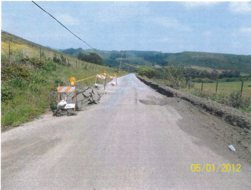
Photo 2. – Photo looking east at roadside and ditch damage caused by the landslide. An asphalt concrete-lined ditch exists to the left of the uplifted pavement and is no longer functioning due to the slide material. Water now moves around and through the distorted pavement.
