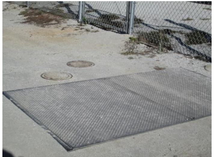
16. View of water and utility plates near the tank enclosure
