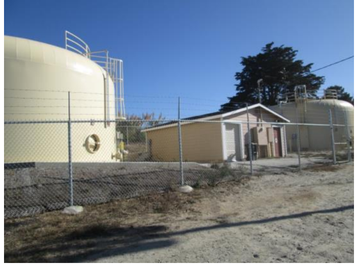
14. View of water supply tanks on the southern corner of the subject property
