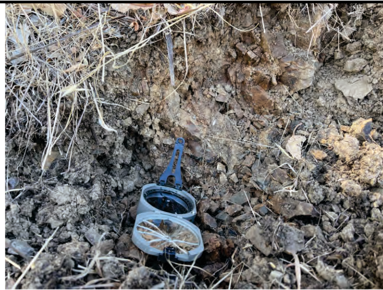
Photo 1b. Exposure of closely jointed shale and graywacke at arrow in Photo 1a.
