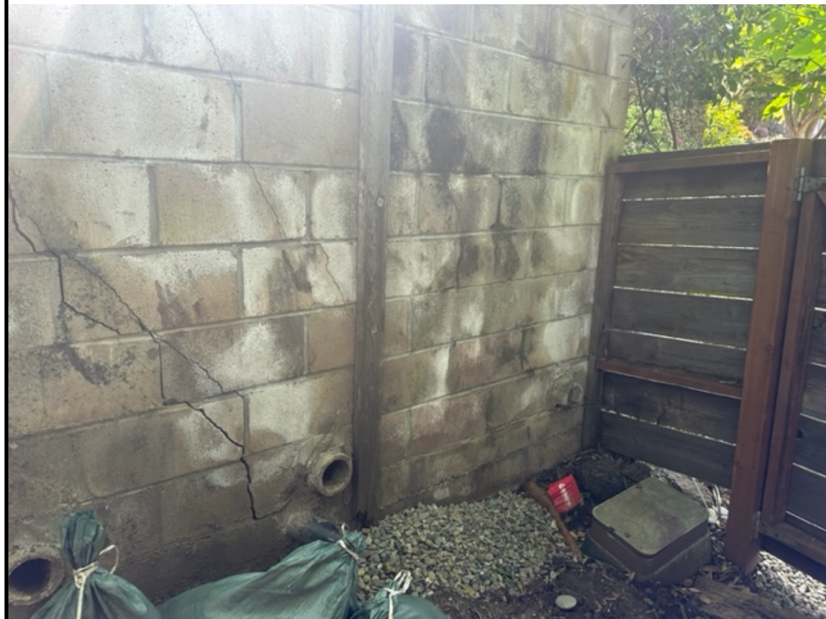
G-3. North view at northwest corner of your property where a make-shift gravel basin and sandbags have been placed in an effort to control runoff evidently derived from wall backdrain discharge during periods of rainfall.
