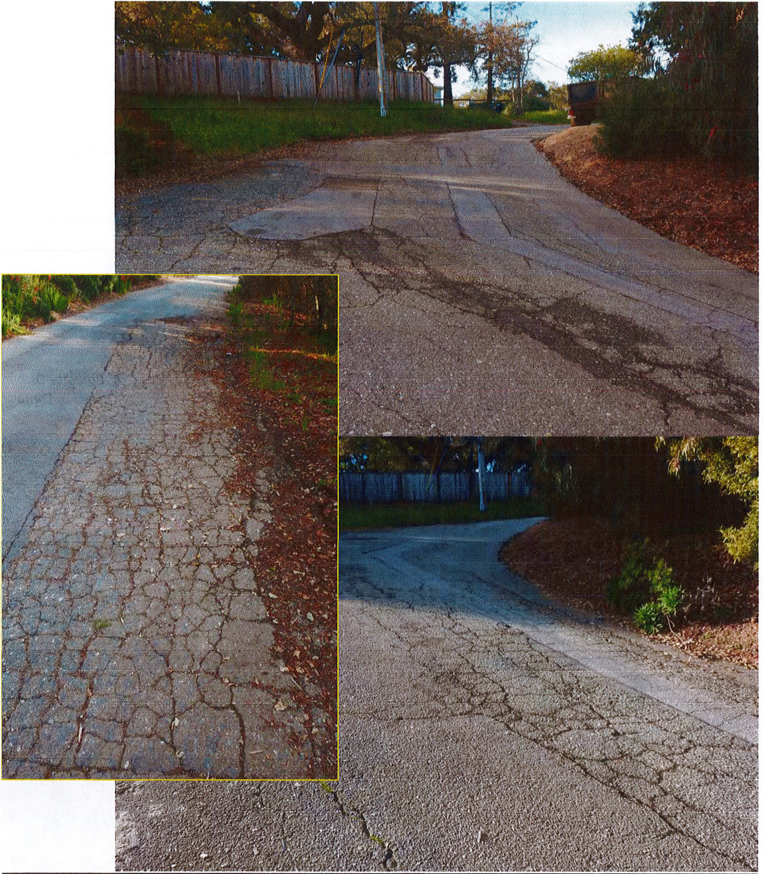
Figure 5. Photos checked and patched asphalt indicating underlying water along Loma Rd, San Mateo County, CA. Photos taken on March 2, 2023.
