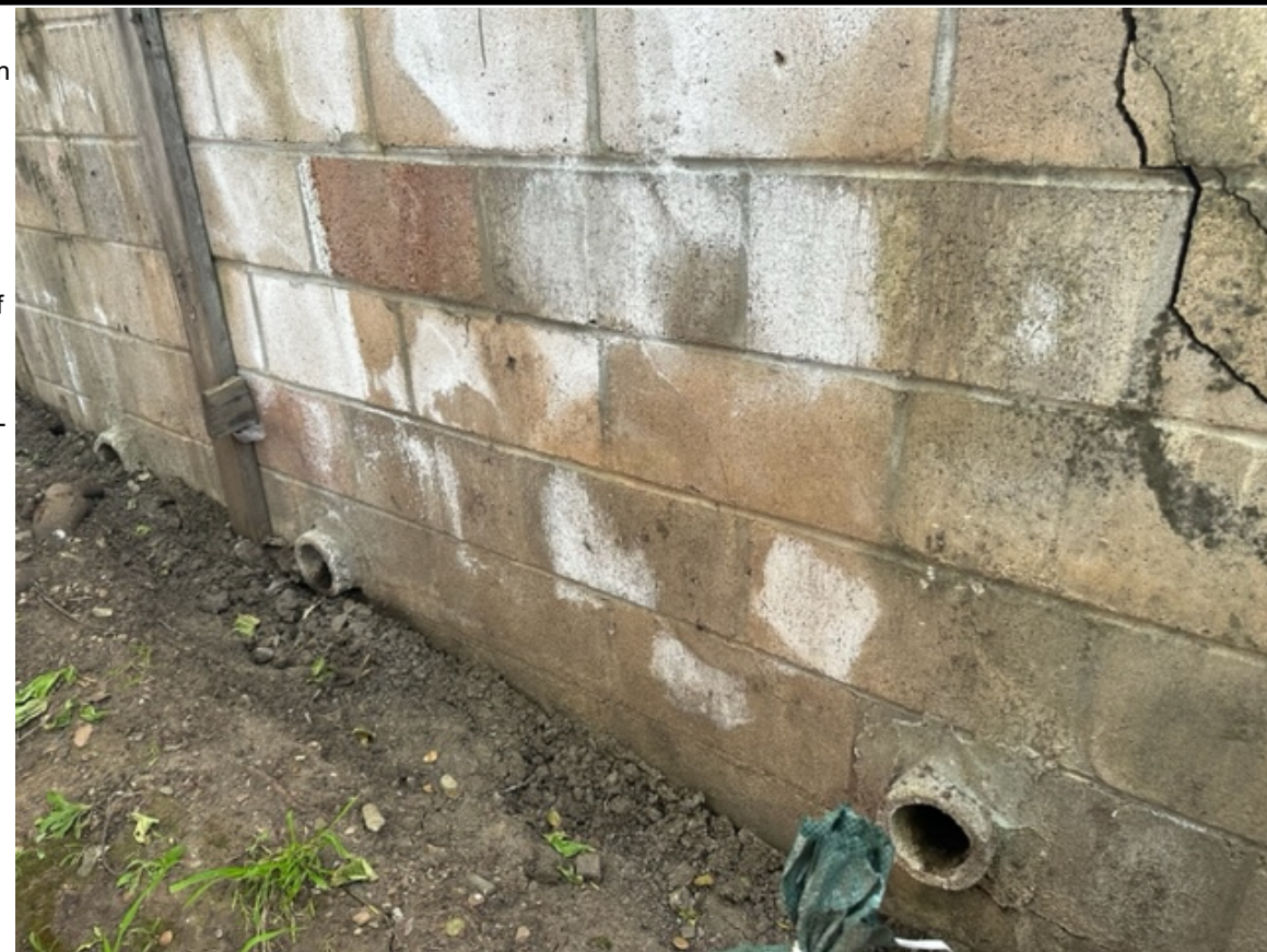
G-3. Southwest view of retaining wall (Photo G-1). Note nature and wetness of the wall face.
