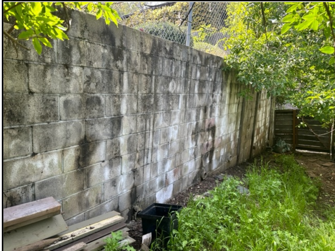
G-1. North view of dilapidated historic masonry retaining wall on 730 Loma Court facing the northwest corner of your property.
